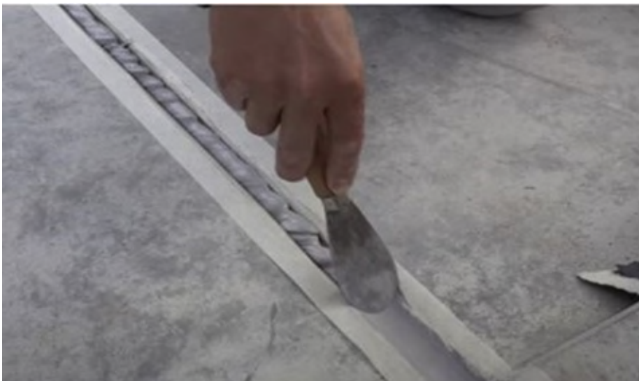
Figure 12 - After filling the joint tool off to create a smooth concave surface and ensure the sealant is filling the joint.
