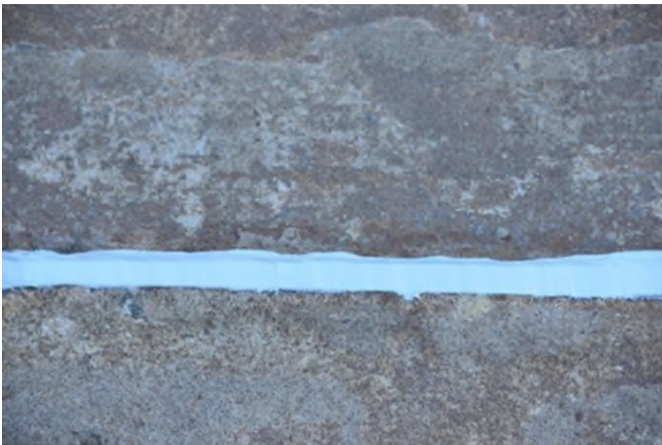
Figure 14 - Leave joint to cure and it is best to apply the sealant when the temperature is constant or rising.
