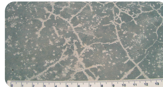
Early age cracks by drying shrinkage
