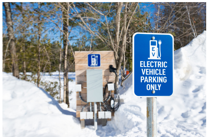
Electric vehicle charging station
