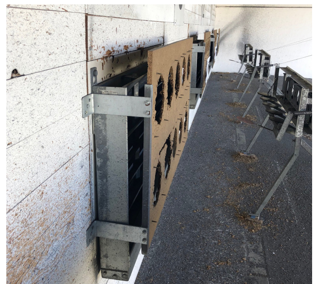
Lead Collection System
