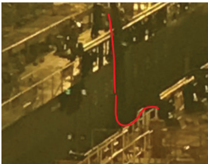
Incorrect lift causing U in hose
