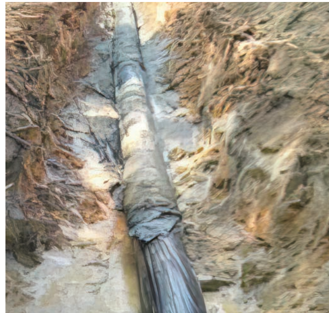
Figure 10: Assembled-line method, pipe built on polyethylene and covered with drilling fluid to facilitate installation
