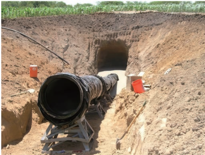
Figure 11: Pipe has been pulled through the bore path, ready to attach to the remainder of the pipeline
