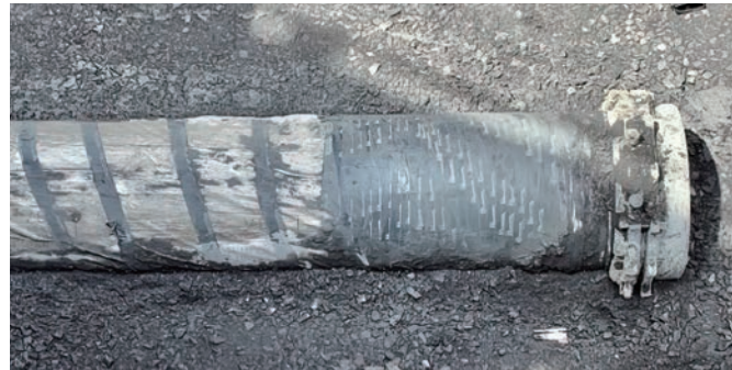
Figure 18: Exposed V-Bio® enhanced polyethylene encasement after HDD installation—Polyethylene encasement uncompromised from installation
