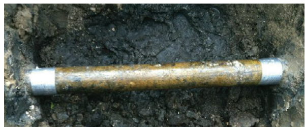
Superficial oxidation of cast iron pipe since 1958
