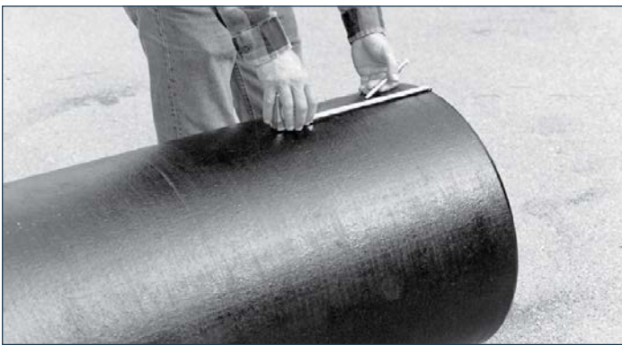
Step 4. Mark the location of the weld-on retainer ring from the cut end of the pipe per the manufacturer's specifications.
