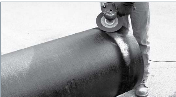
Step 5. Remove the pipe's asphaltic coating on the area where the retainer ring will be welded with a solvent wash or by burning with a torch; then grind the retainer location to bright metal.
