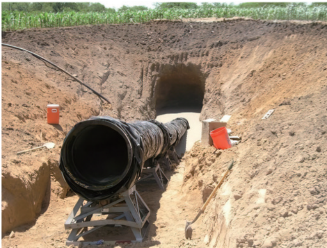
Figure 11: Pipe has been pulled through the bore path, ready to attach to the remainder of the pipeline
