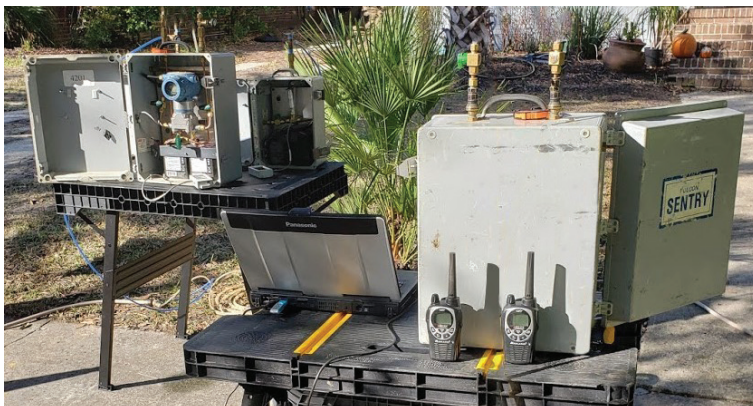
Figure 2: Sentry flow meters used to measure velocity and headloss. On the right is the representative profile of turbulent flow in a pipeline.
