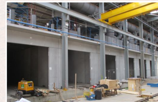
Energy efficient dryers at Ellistown project
