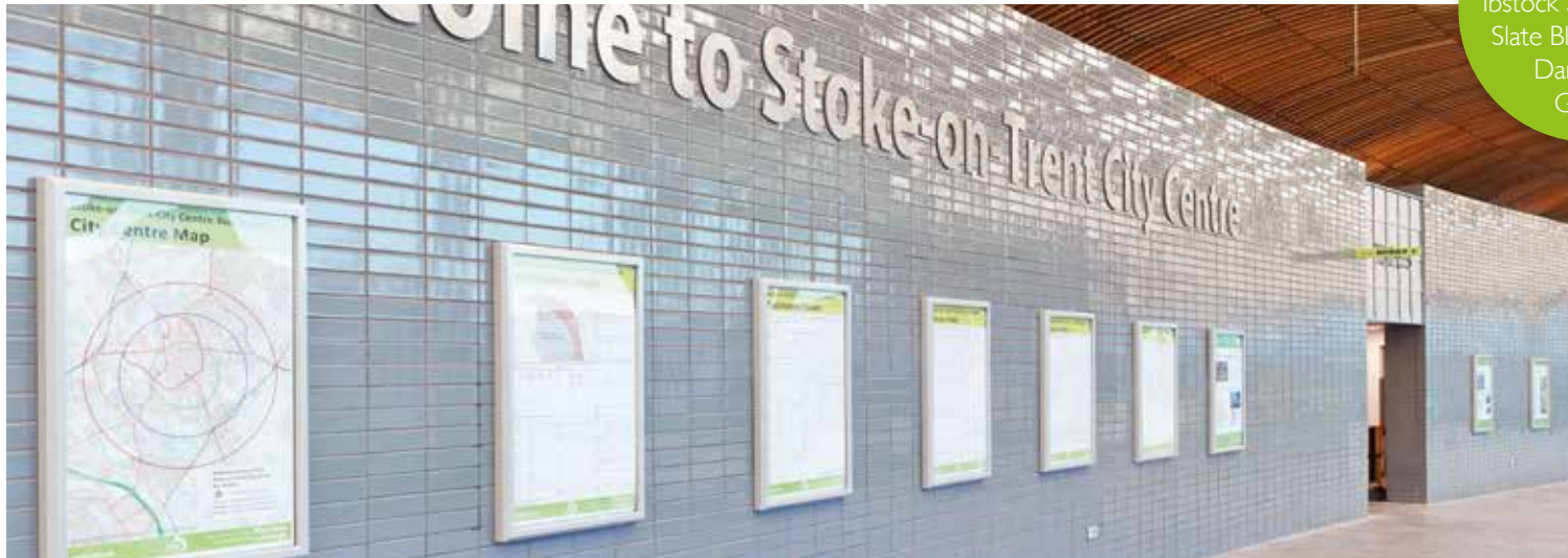
Dark Grey Glazed bricks are laid stack bonded for a modern visual effect.
