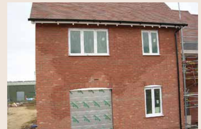
This building was subject to a period where no waterproof protection was in place before roof construction was completed.
