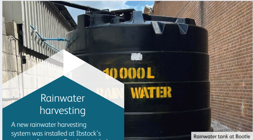
Rainwater tank at Bootle
