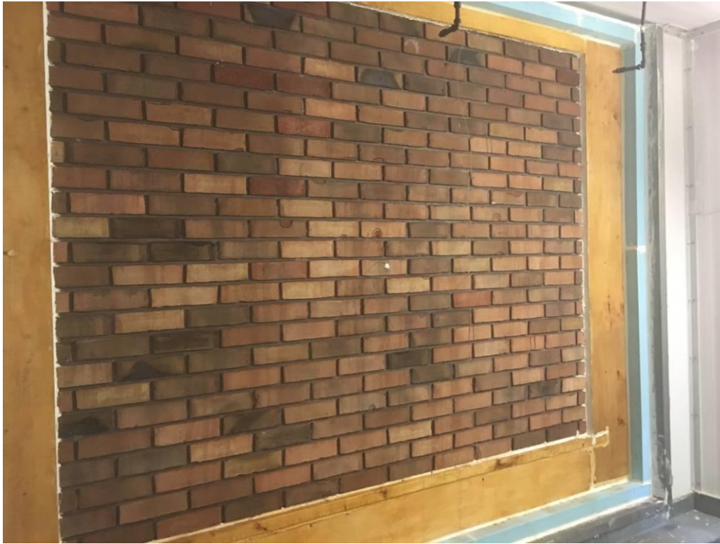
Plate 5 - Front of Panel after Test
