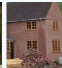
A missing down-pipe can cause permanent saturation staining.
