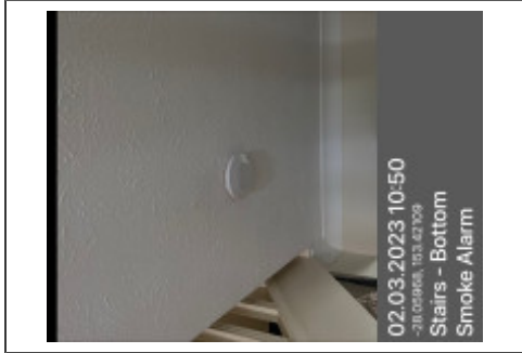
RFC - Stairs - Bottom (GF/Entrance) Exp. Date: 4/2030
