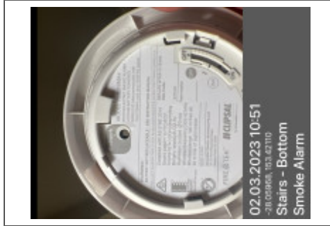
RFC - Stairs - Bottom (GF/Entrance) Exp. Date: 4/2030
