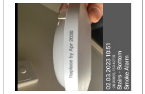
RFC - Stairs - Bottom (GF/Entrance) Exp. Date: 4/2030
