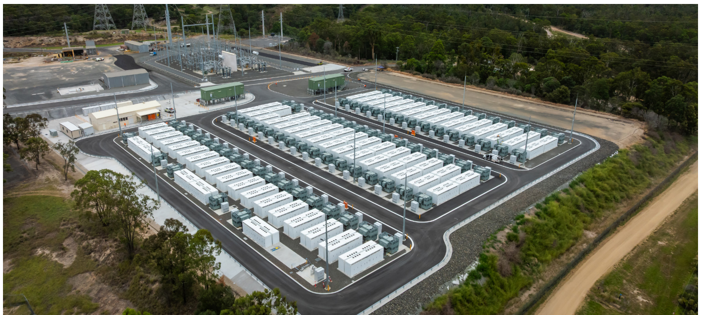
The battery is located onsite at Tarong power stations.
