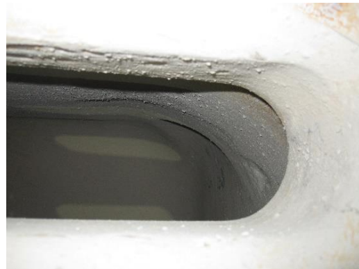
Figure 7 – High Concentrated Wear in the Discharge End Outer Pulp Lifter
