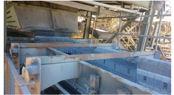
Discharge Chute Including Skirt Liners
