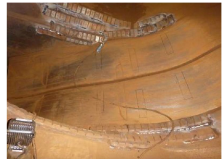
Worn AR Steel Liners with repairs
