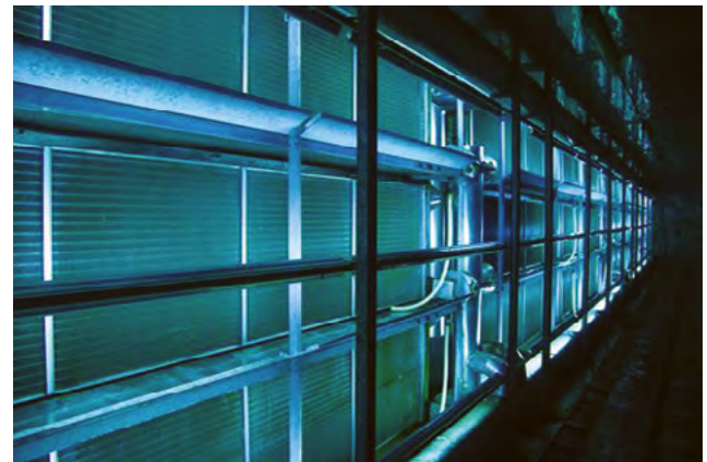
UVGI system, Alphaa UV
