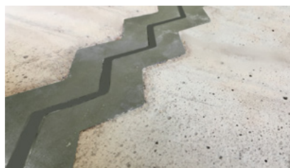
Joint expansion after shrinkage
