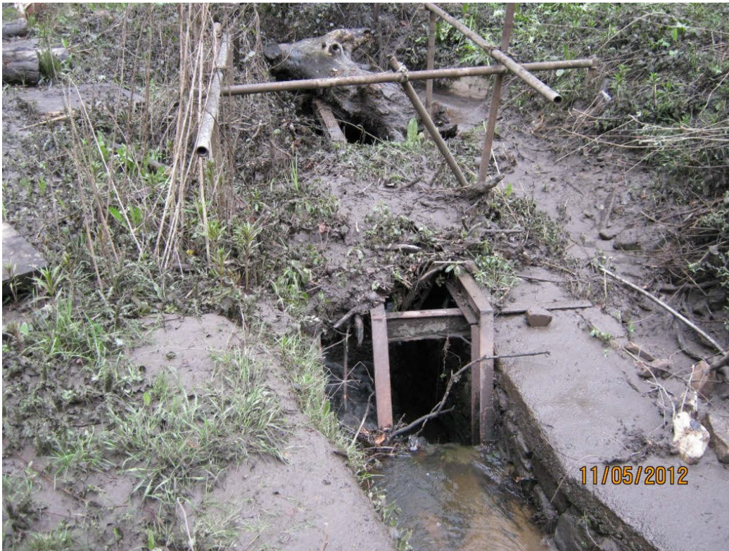
Figure 6: Partially blocked inlet trash screen (Source: SMBC Highway Structures)
