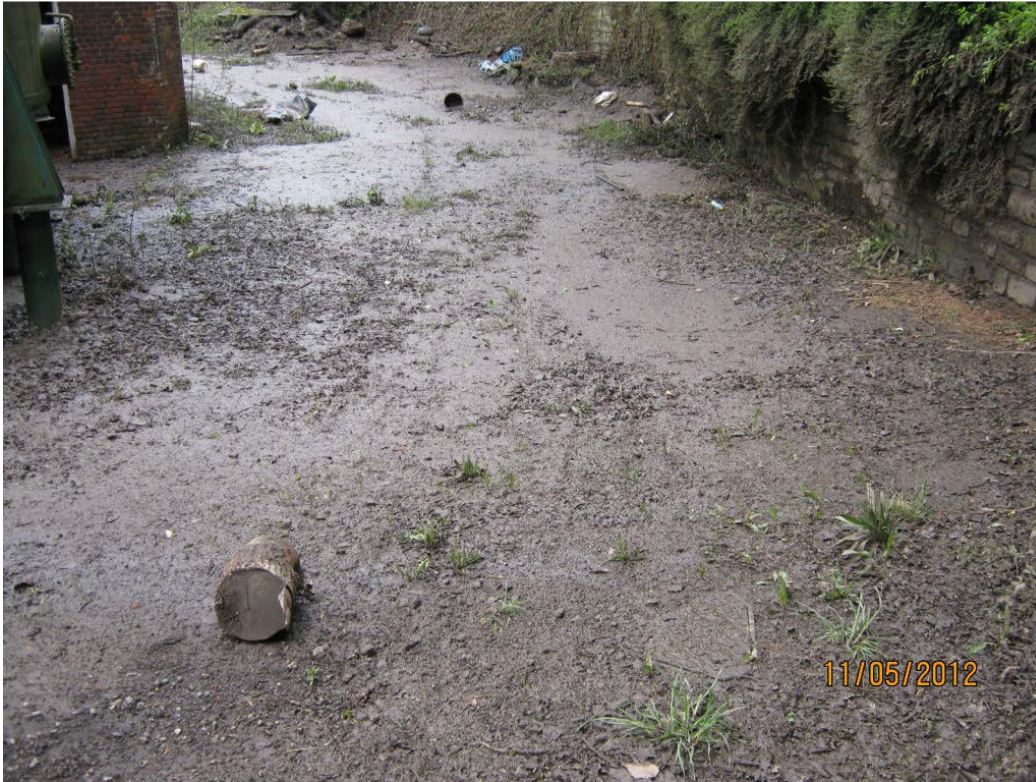
Figure 5: Flooding photograph (Source: SMBC Highway Structures)
