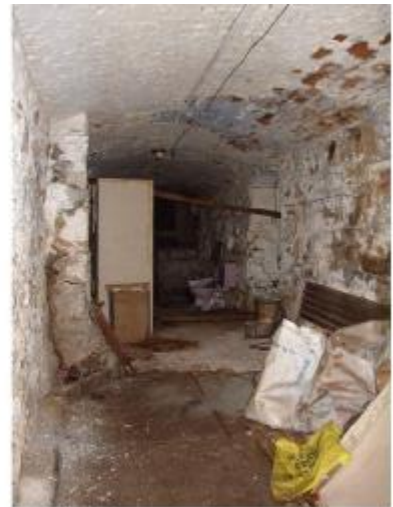
Part of the below ground culvert system which connected to the Lily Wheel
