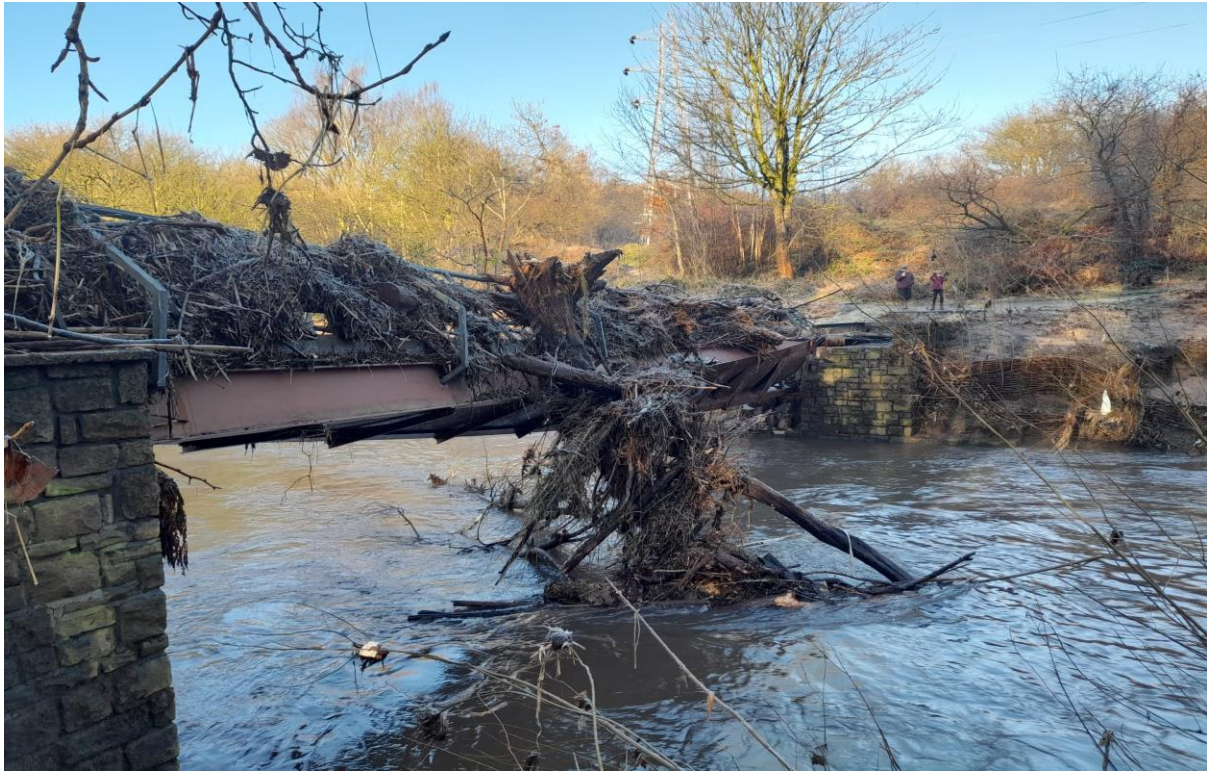
Figure A7.3. Bridge badly damaged in Reddish Vale Park.
