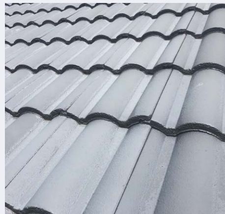
Does your roof appear faded or dull? Environmental fallout such as salt residue, dirt or dust deposits can cause this aesthetic change.
