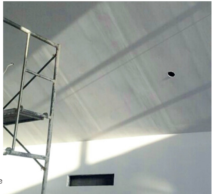
Example of Level 4 Finish with a critical light problem
