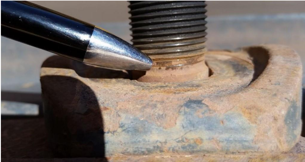
Figure 2 - UNACCEPTABLE stud and clamp combination, the stud thread ends above the nut seating surface of the clamp.
