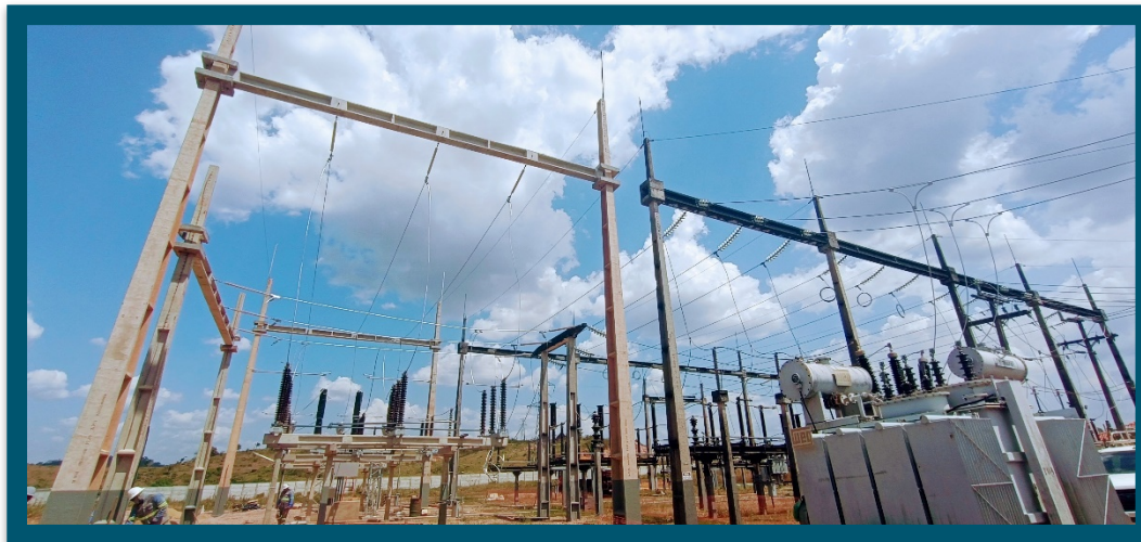
Figure 3 – Novo Progresso Substation
