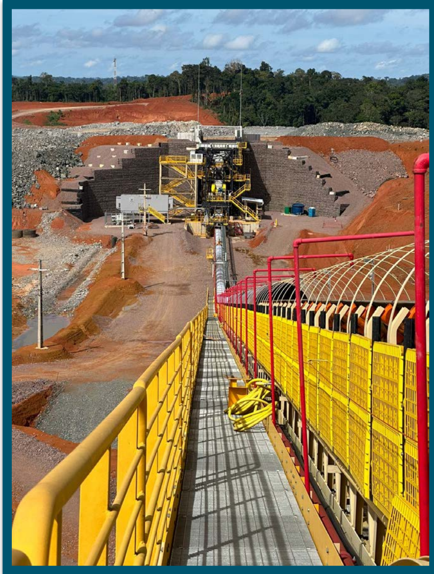
Figure 4 – Primary Crusher and Stacker Conveyor
