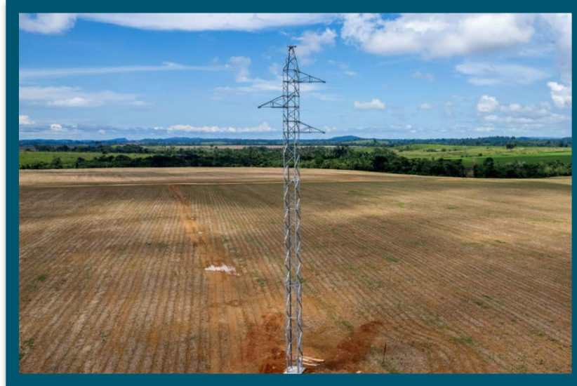
Figure 8 – Transmission Line Tower
