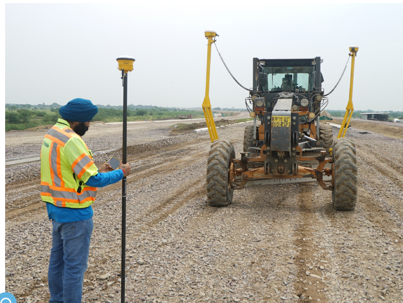
The Trimble GCS900 3D Grade Control System guiding a Case motor grader and the SPS986 Site Positioning System to check the grade.
