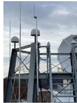
Figure 20. Antenna installation of LDACS ground station installed in Oberpfaffenhofen
