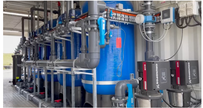
Infinite Water Hydroxon™ Catalytic Oxidation Reactors
