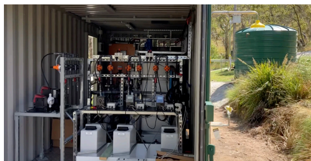
IW's NPWS Water Treatment Plant
