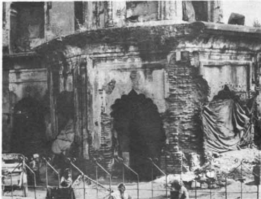
126 Lucknow Rumi Darwaja : South Bastion western facade before conservation. See page 219
