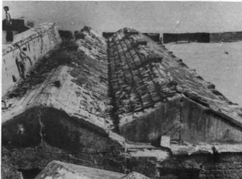
136. Fort St. Angelo, Cannanore : Showing the leaky terrace of the horse stables before conservation. See page 223
