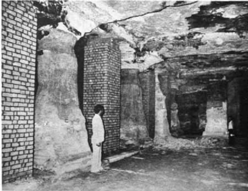
96 Bagh Caves : General view of the row of Decayed pillars in Cave 2. before conservation. See page 205
