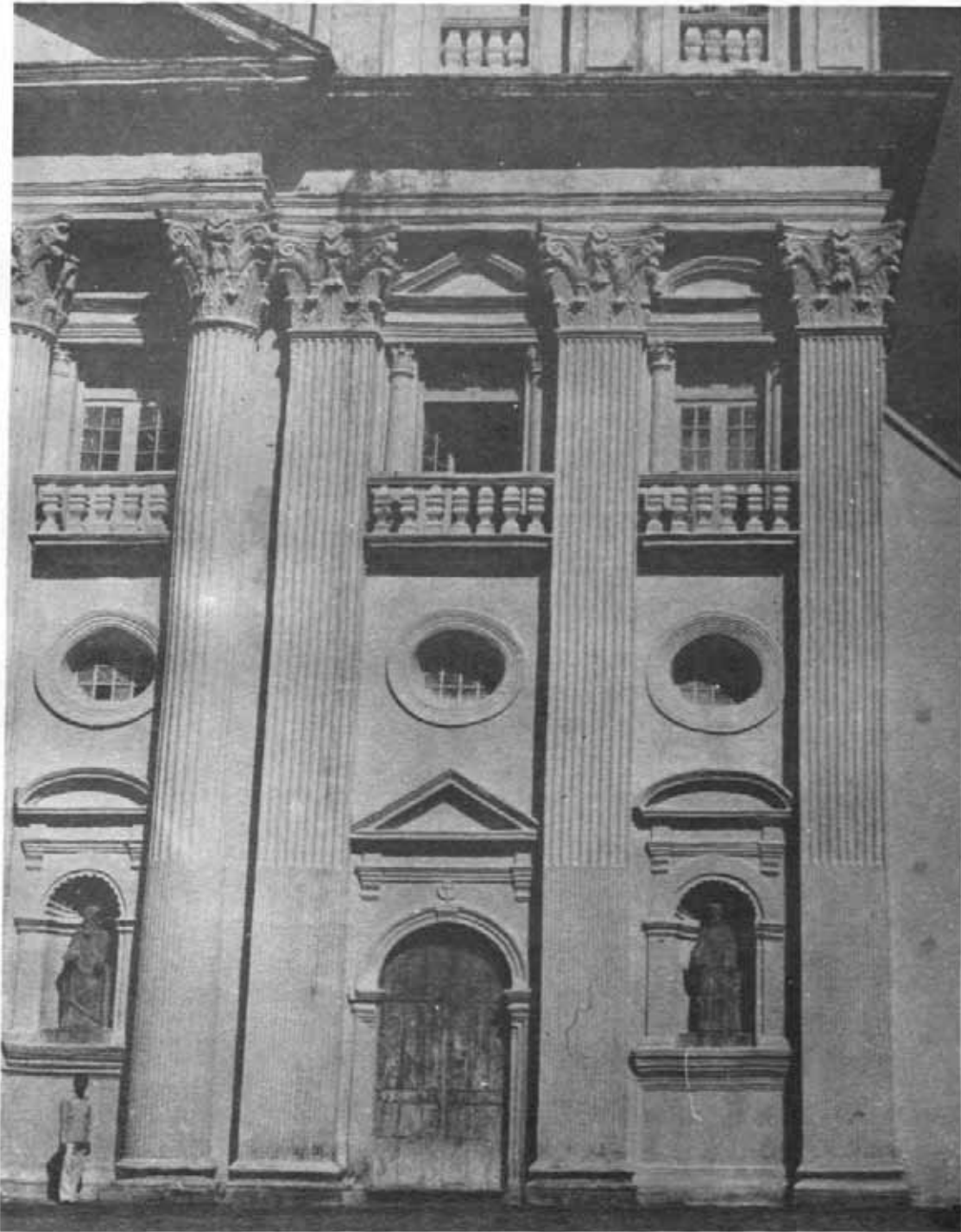
163 St. Cajethan Church : Close up of the part of facade from west after conservation, See page 227
