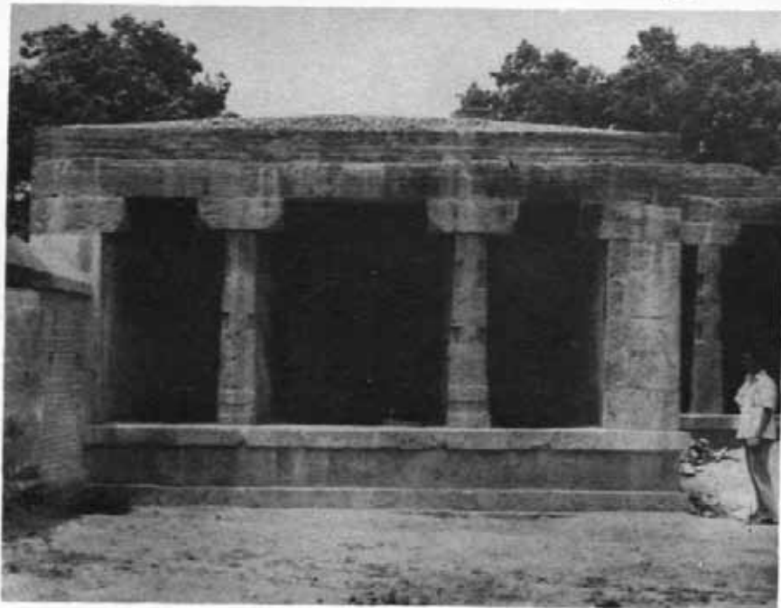
151 Venkatesa Perumal temple, Tirumukkudal : View showing before the removal and re-erection of Anjaneya subshrine after conservation. See page 225
