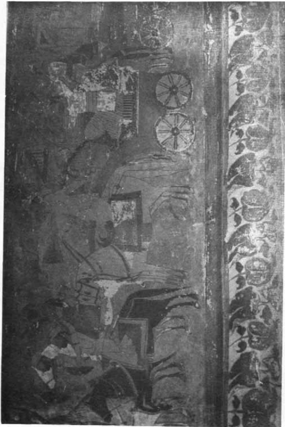
183 Sujanpur Tira : Painting on the wall of the verandah of Narbadeswar temple before chemical treatment. See page 242
