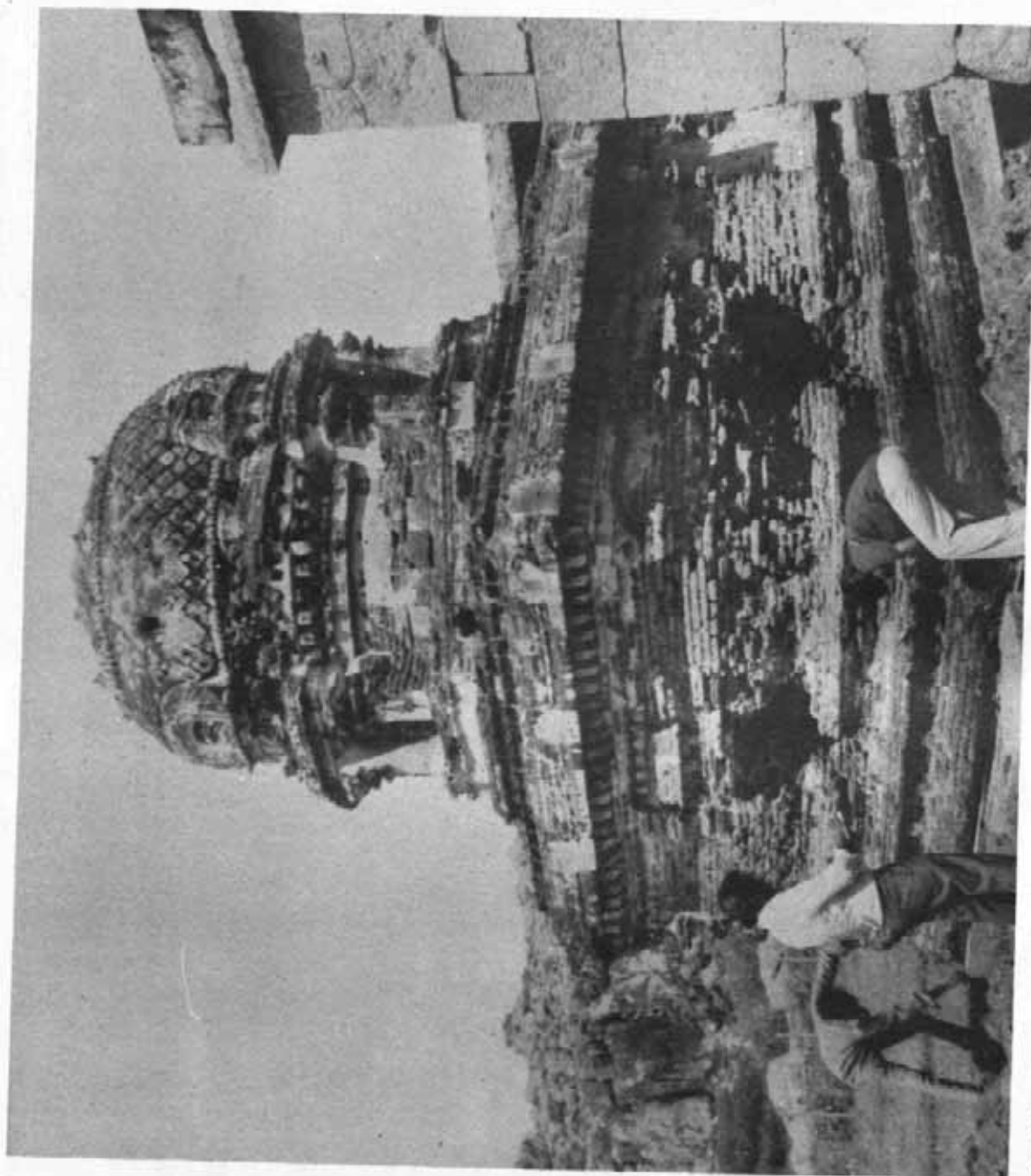
146 Siya Manglam Rockcut cave temple : View showing the art of plumb portion of the Ganesh Shrine before conservation. See page 224
