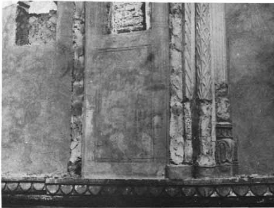
124 Asaf-ud Daula's Imambara, Lucknow : Southern facade of 1st entrance gateway before conservation. See page 218
