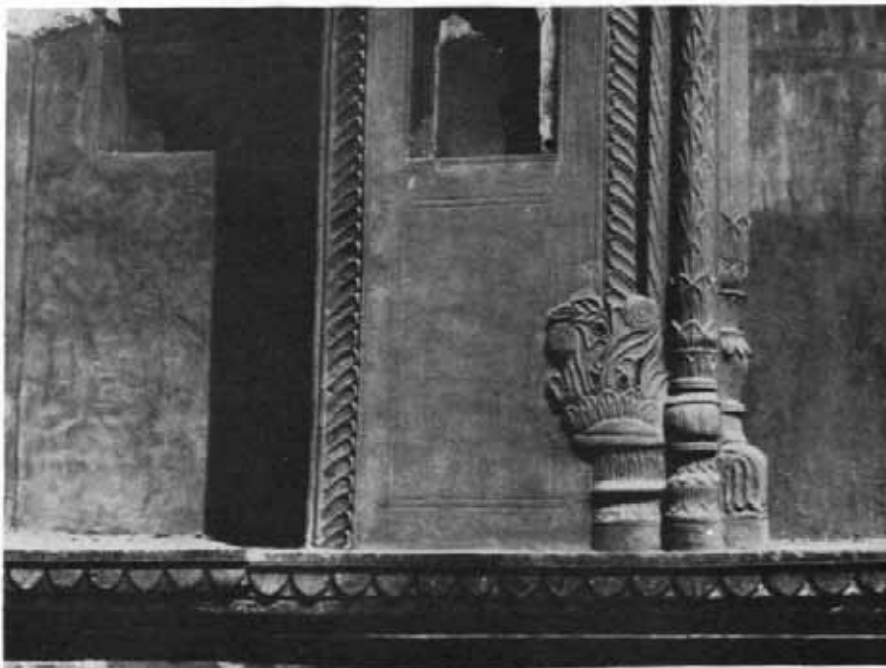
125 Asaf-uD Daula's Imambara, Lucknow : Southern facade of 1st entrance gateway after conservation. See page 218
