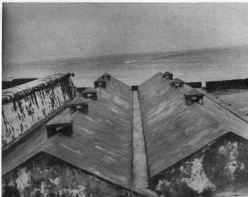
137 Fort St. Angelo, Cannanore : Showing the leaky terrace of the horse stables after conservation See page 223
