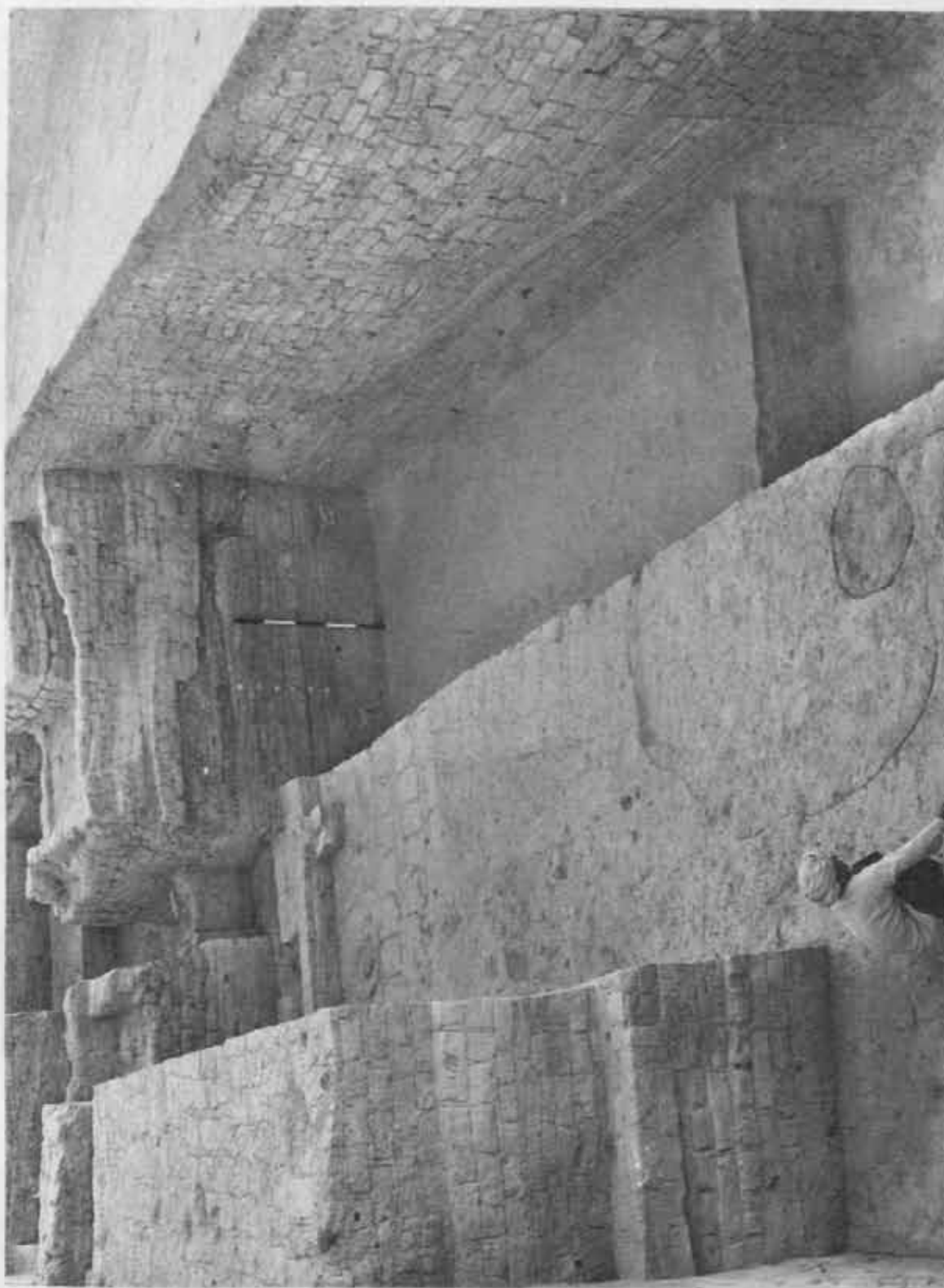
Banawali : exposed pre-Harappan and Harappan defences and other structural phases, view from north. See p. 23
