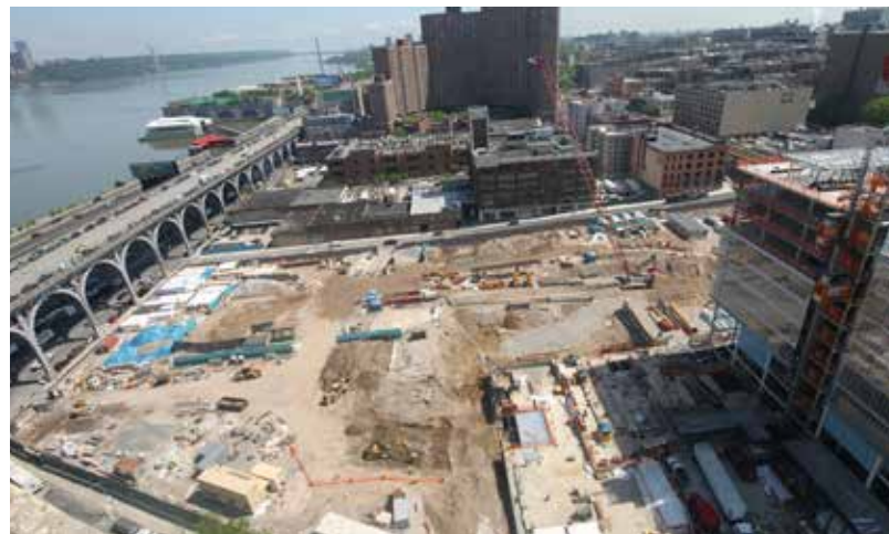
Manhattanville campus under construction: at right Jerome L. Greene Science Center; at center is outline of Lenfest Center for the Arts
