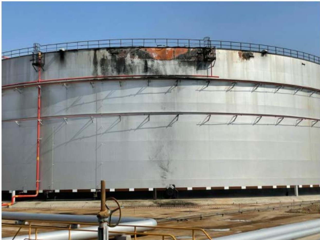
Diesel storage tank damaged by Houthi missile strike on Aramco depot in Jeddah
