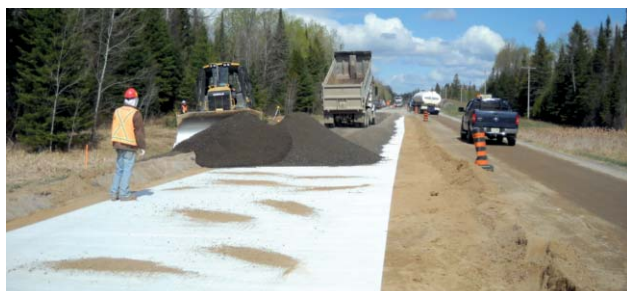
Fig. 9 Combigrid® used over a soft subgrade to achieve soil reinforcement and soil separation and filtration to ensure long-term performance
