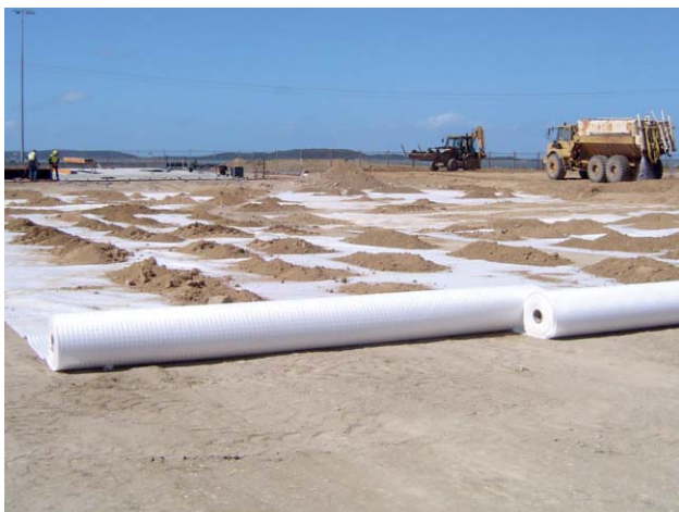
Fig. 3 Combigrid® installed as base course reinforcement where multi-directional stiffness is of great importance
