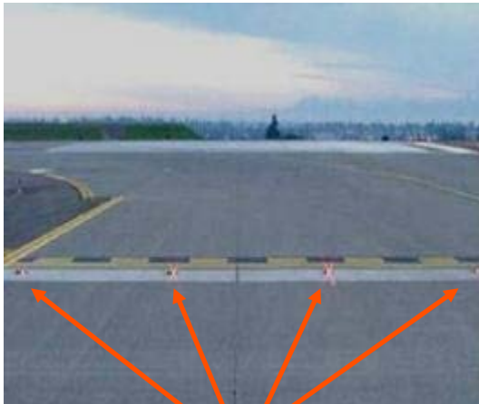
In-Pavement Runway Guard Lights
