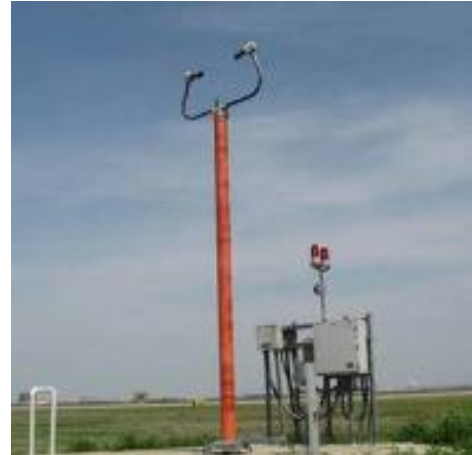
Runway 17C/35C mid-point Transmissometer RVR tower
