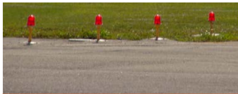
Denied Area / No Entry Lights
