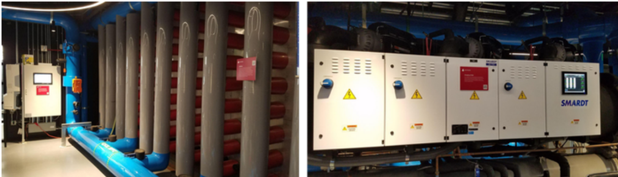
Figure 11. The pipes leading to the IceBricks and the charging chiller.
