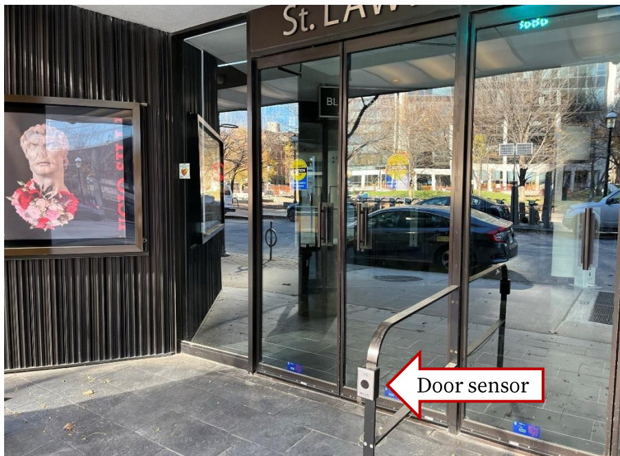
This picture shows the automated doors and wave-to-open sensor for our building.
