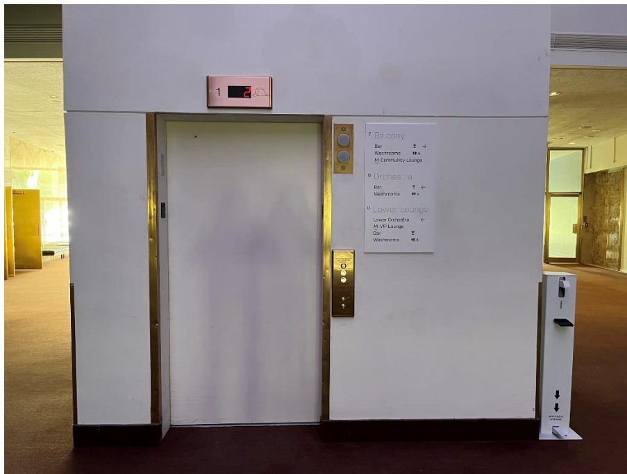
This picture shows the elevator in the main lobby.
