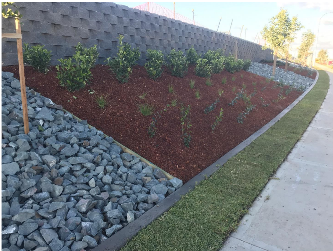
Figure 6: Example of retaining wall in location of fill adjacent to road reserve
