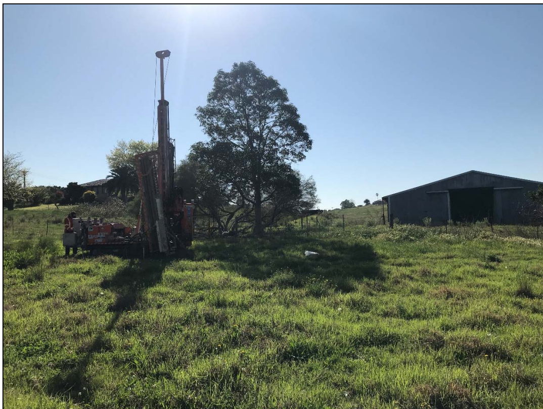
Figure 4 – General site overview and drilling rig setup in the location of BH1
