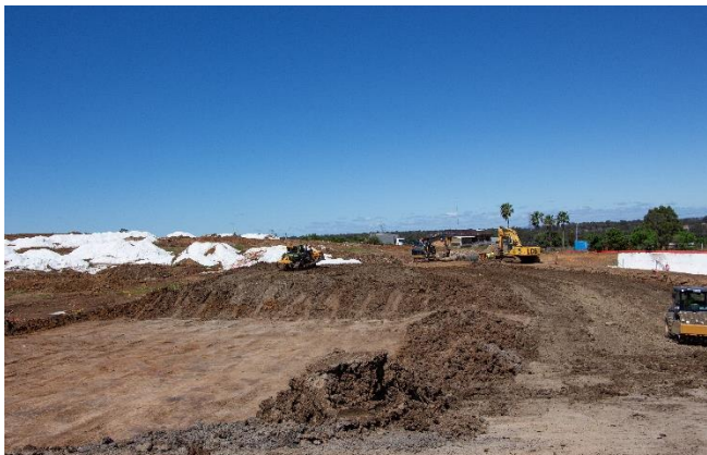
Figure 4 View of Westlink Stage 1 Lot 4 from the Abbotts Road extension looking south
