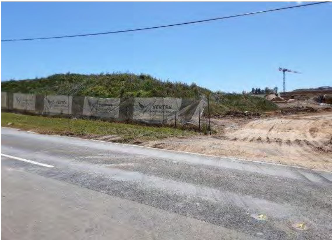
Photo 21 Disturbances along Aldington Road: fencing and stockpile of soil associated with construction, facing north-east
