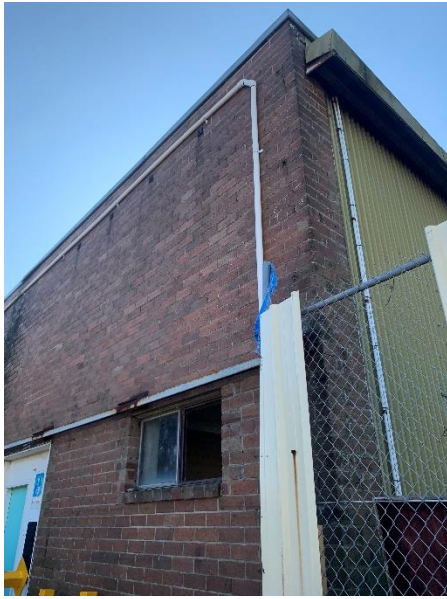
Figure 33. Junction between western and southern facades, noting change in material (Source: Artefact, 2022)
