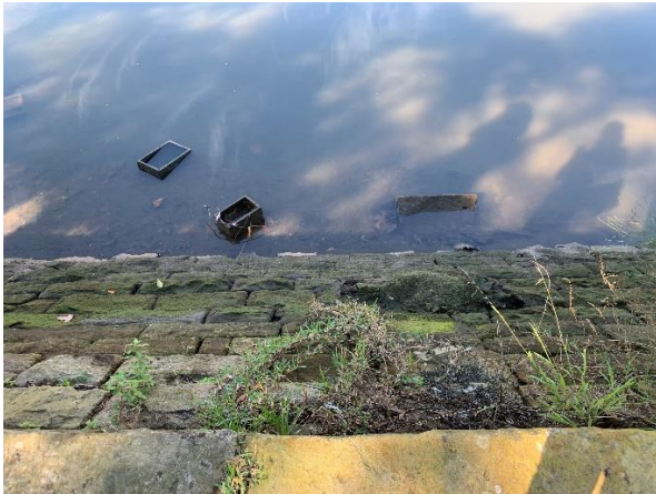
Figure 58. Alexandra Canal sandstone wall from 28 Burrows Road showing existing stormwater outlet (Source: Artefact 2022)
