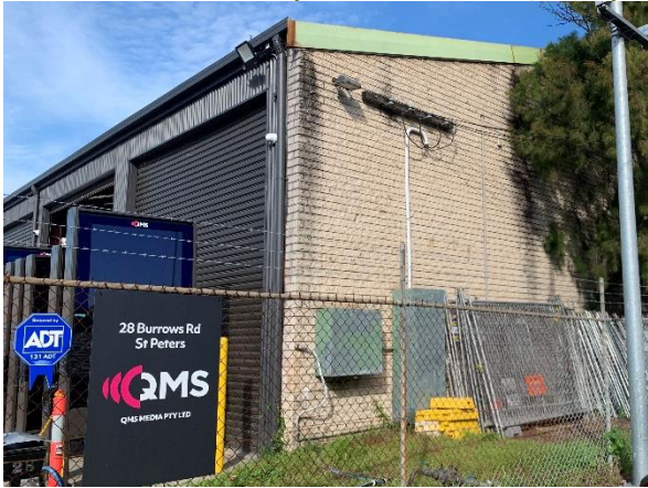
Figure 38. Detail of warehouse, looking south from Burrows Road. Junction of north and east façades. (Source: Artefact, 2022)
