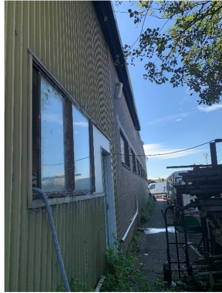
Figure 28. Southern façade, looking east. Note the change in material from corrugated iron to brick. (Source: Artefact, 2022)
