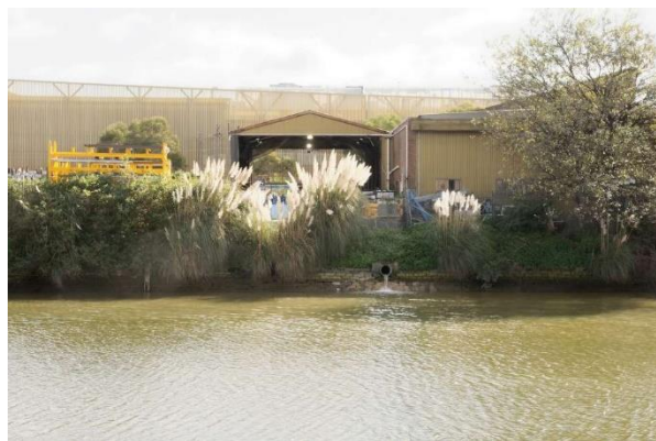
Figure 63. Canal wall adjacent to 30 Burrows Road, showing another storm water outlet, which has been releasing acidic drainage indicated by the lack of algae. (Source: LOGOS, 2022)
