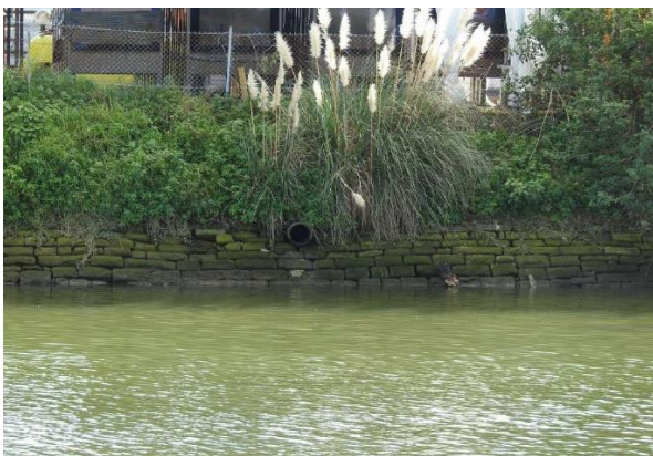
Figure 62. Stormwater outlet adjacent to 28 Burrows Road, view from the eastern bank (Source: LOGOS, 2022)
